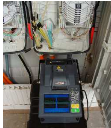
Fig. 9 Illustration of field installation. In the foreground, a splicing machine and, in the background, a connection box.
